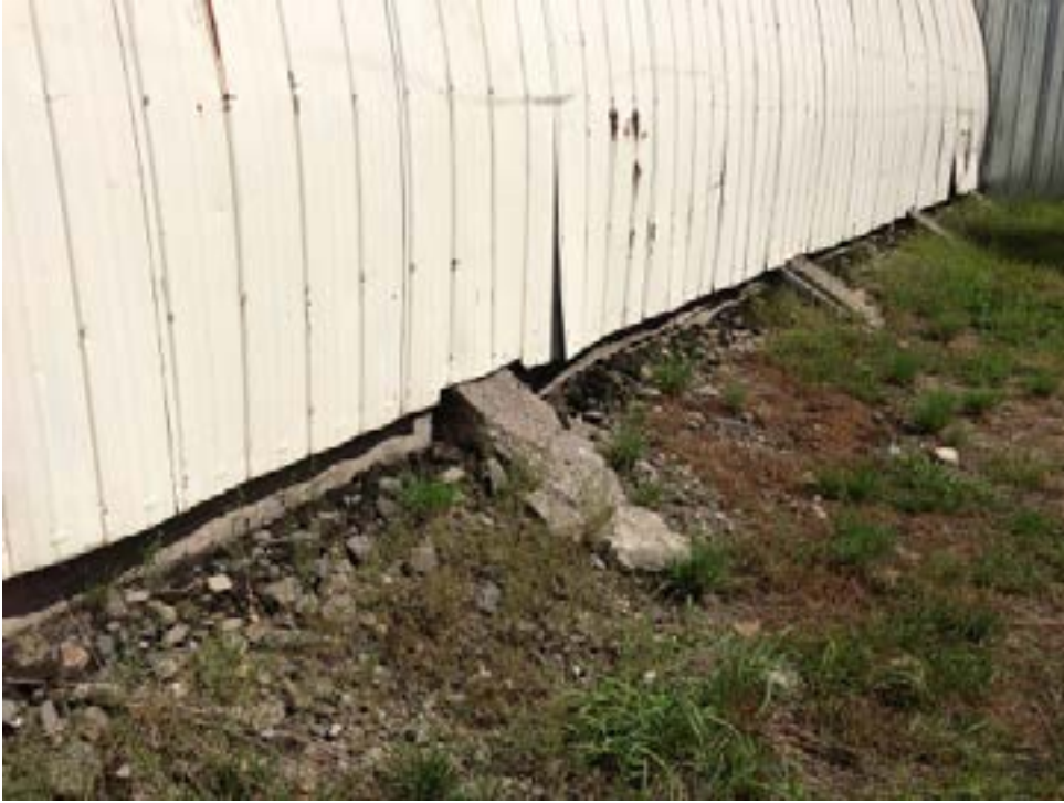
A3/S1 structural buttress supports are damaged
