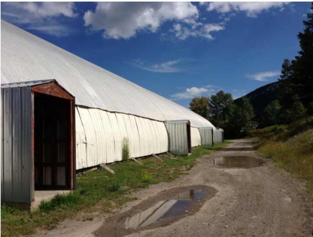
C4 - Fire lane access requires regrading and a swale to keep spring runoff from Mountain away from the building foundation
