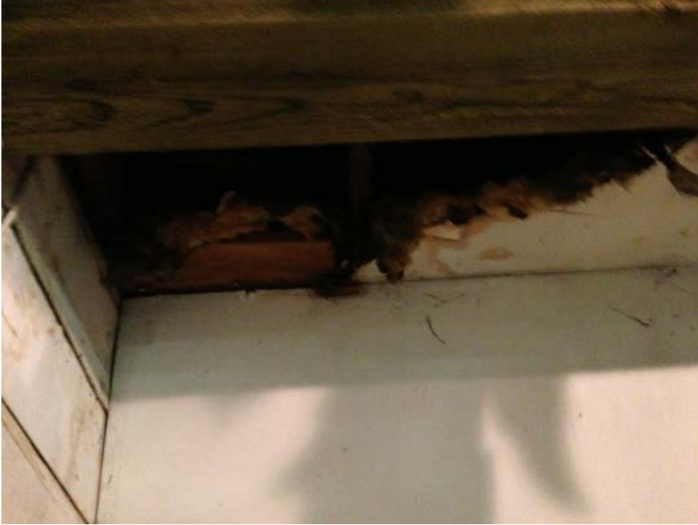
A7 - Roof taking on moisture
