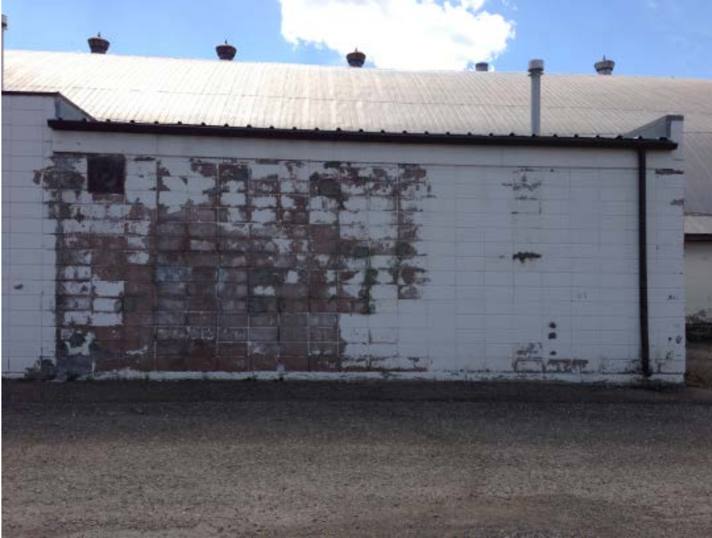
A11- Load bearing block wall damage
