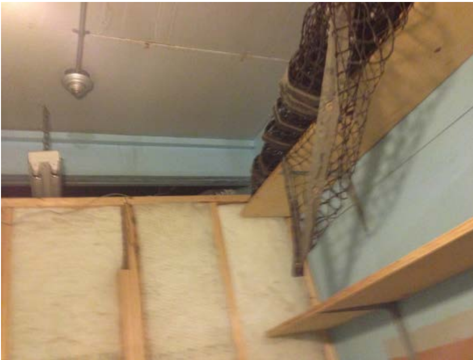
A16 - Fire rating for storage room and electrical room walls are not provided
