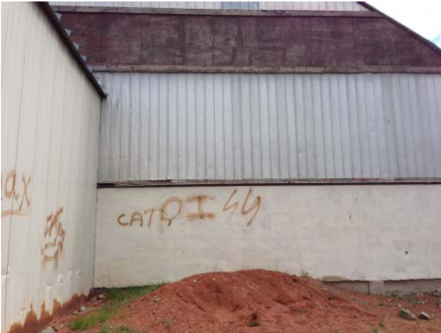
C2- Remove debris and materials from around the building to improve drainage.
