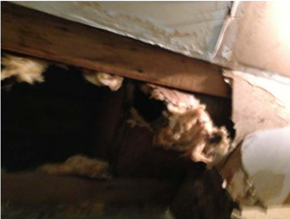
A8 - Roof requires removal and repair
