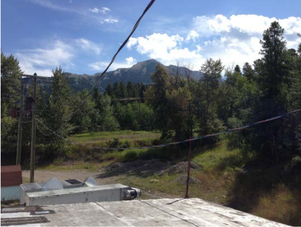
E1 - Live wires are accessible to the roof access
