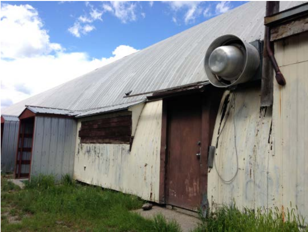
A4- Envelope deficiencies
