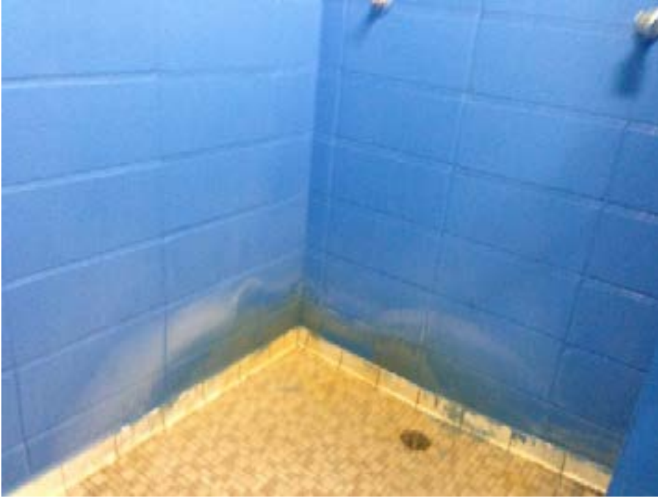
A15 - Change room shower floor tile and concrete block walls are showing damage from moisture infiltration to loadbearing block
