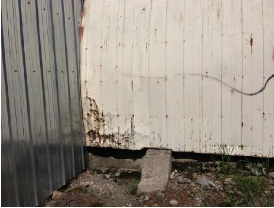
C1- Regrading is required around the building to provide proper drainage
