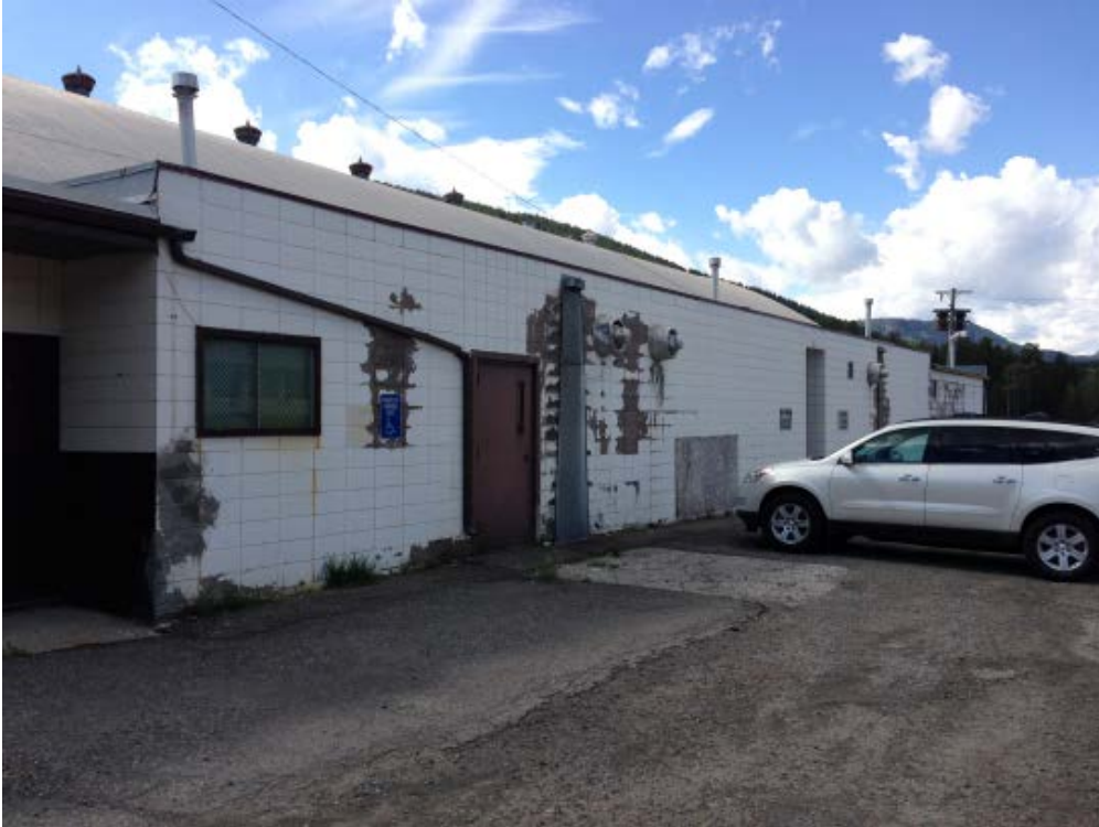
C3 - Paving requires to be replaced and regrading
