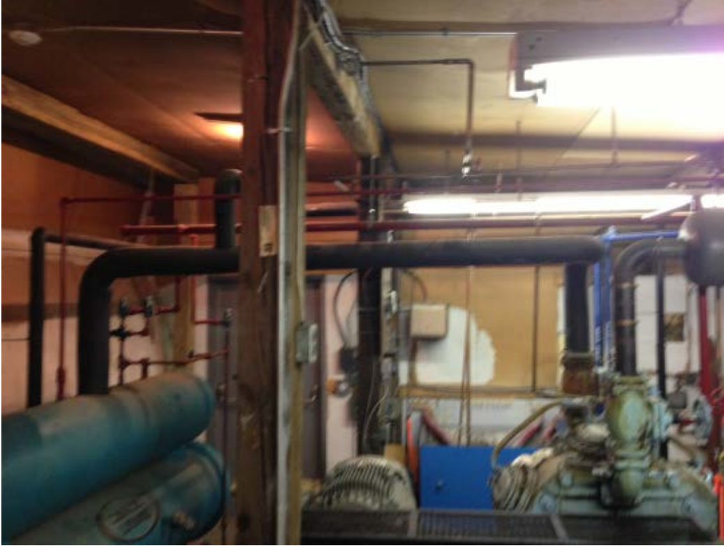
M1 - Ice plant system require to be removed
