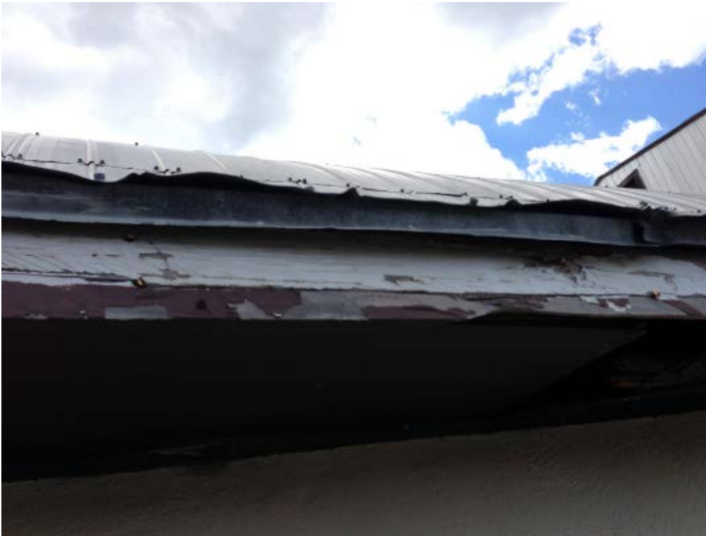
A10- Eavestroughing required control water and snow
