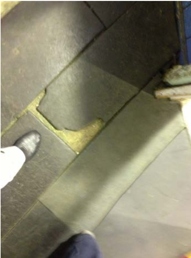
A13and 14 - Indoor skate tile is worn and requires replacement
